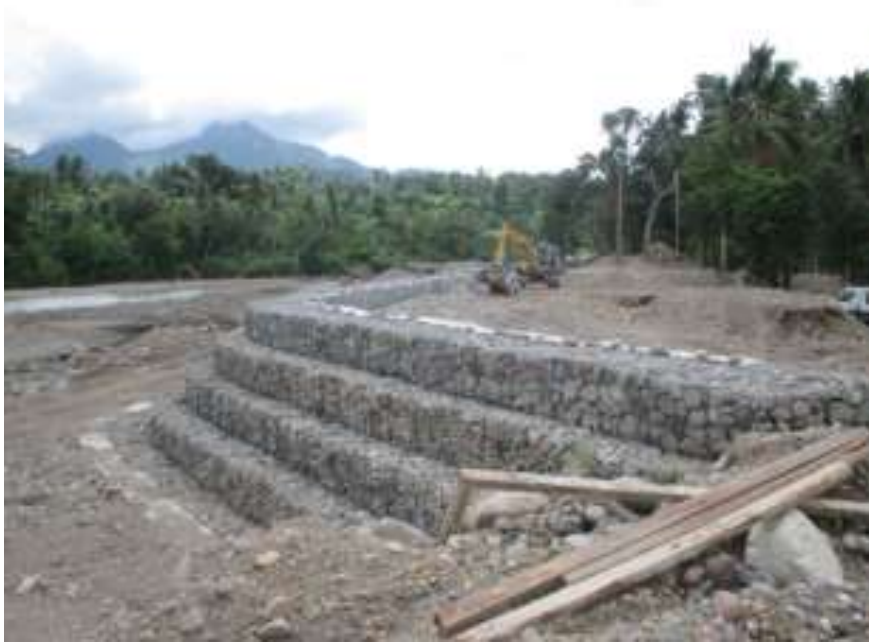
SHORT TERM MITIGATION BEING IMPLEMENTED BY LMWD BASED ON BE SECURE'S DESIGN
