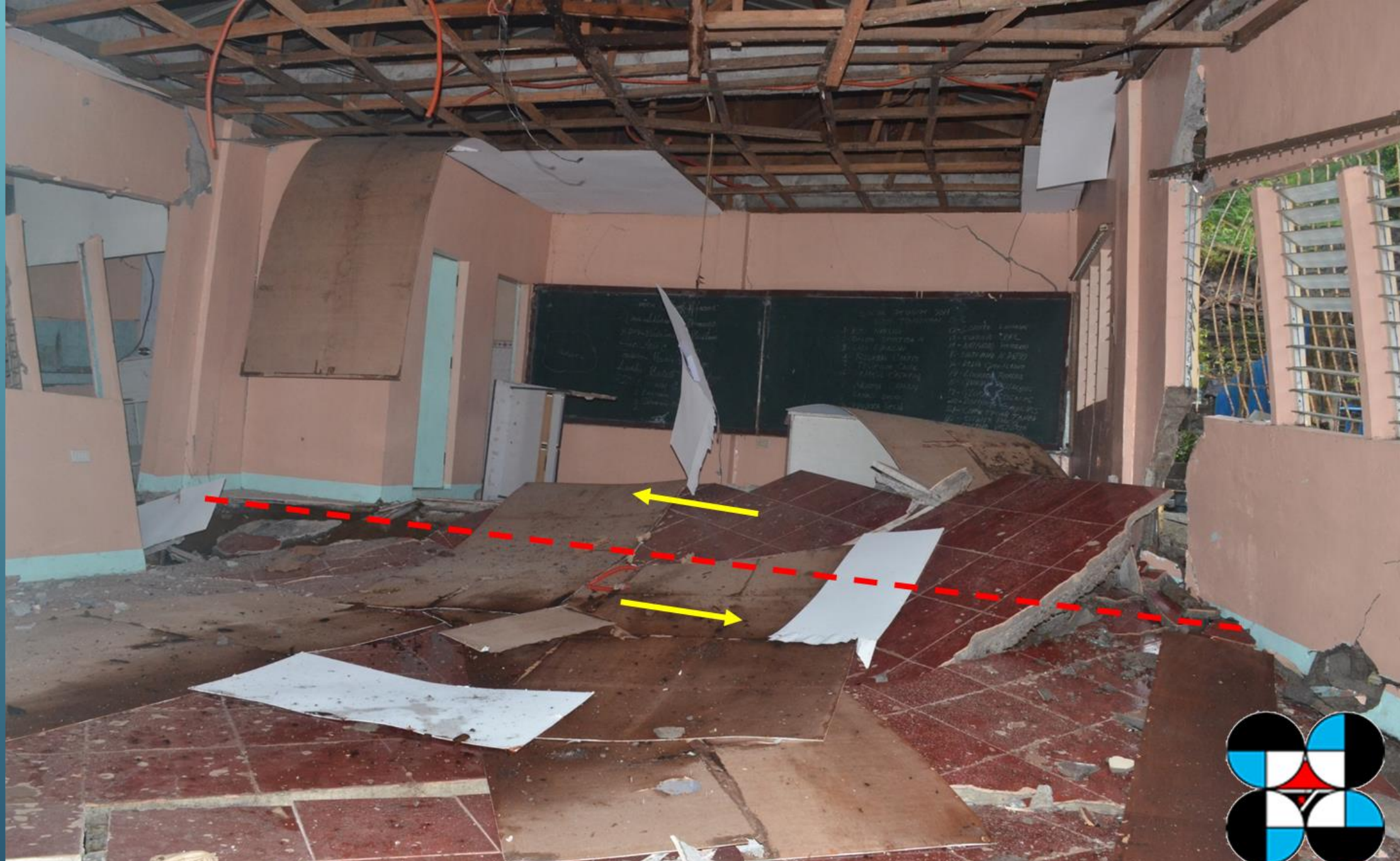
Surface rupture of the 06 July 2017 M6.5 Leyte Earthquake
