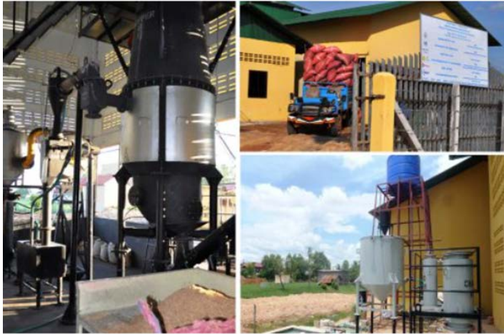
Rice Husk Gasification to Electricity Generation, Cambodia
