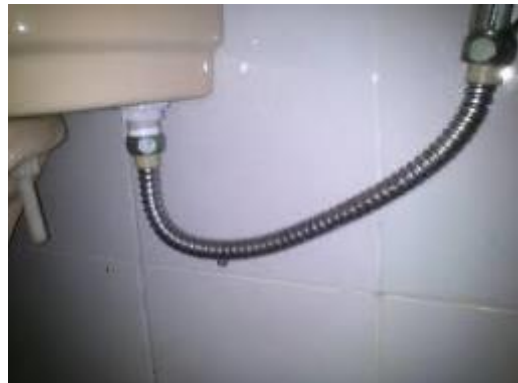
WATER LEAK AT THE CONNECTION HOSE
