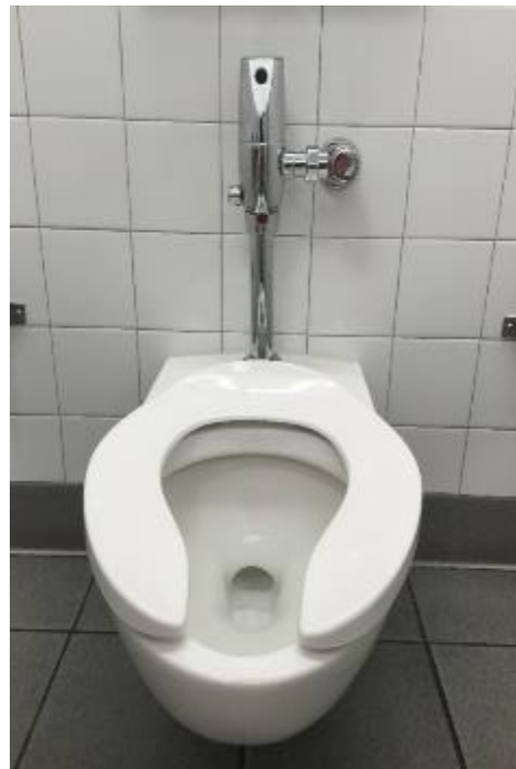
SENSOR ACTIVATED FOM VALVE TOILET
