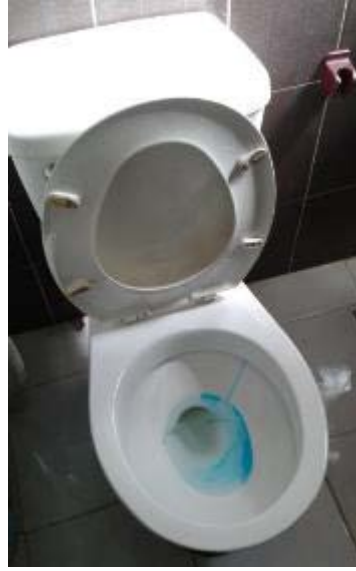
TOILET WITH LEAK AFTER DYE TEST
