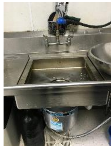
SINK WITH FOOD DISPOSAL GRINDER
