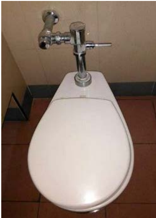
MANUALLY ACTIVATED FOM VALVE TOILET
